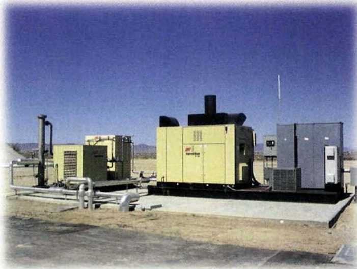
At this California wastewater treatment plant, the installation of an Ingersoll-Rand MT250 microturbine lowered electric costs from about 11 cents/kWh to 4.3 cents/kWh, achieving an annual savings of $225,000. Photo courtesy of Ingersoll-Rand.
